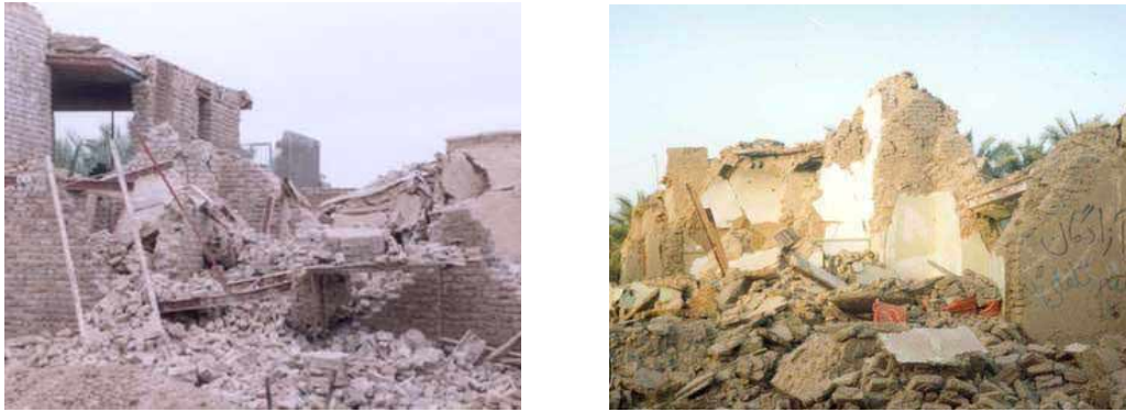
Figure 1. Iran earthquake, 26 December 2003. Collapse of vernacular houses in the city of Bam. ( www.ngdir.ir )
