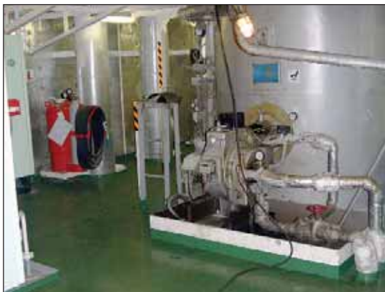
FIGURE 3: Oil burner unit
