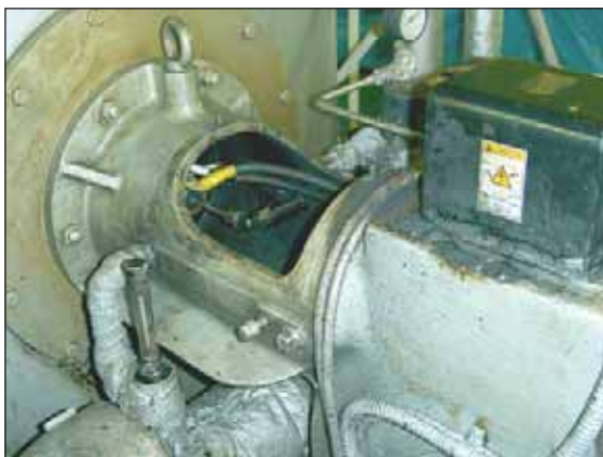
FIGURE 4: Oil burner maintenance opening
