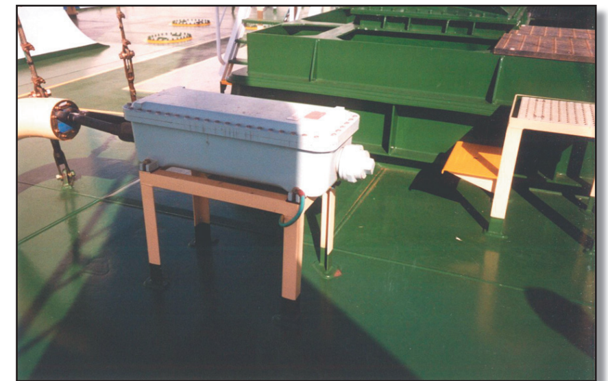
Emergency Cargo Pump Electrical Terminal Box
