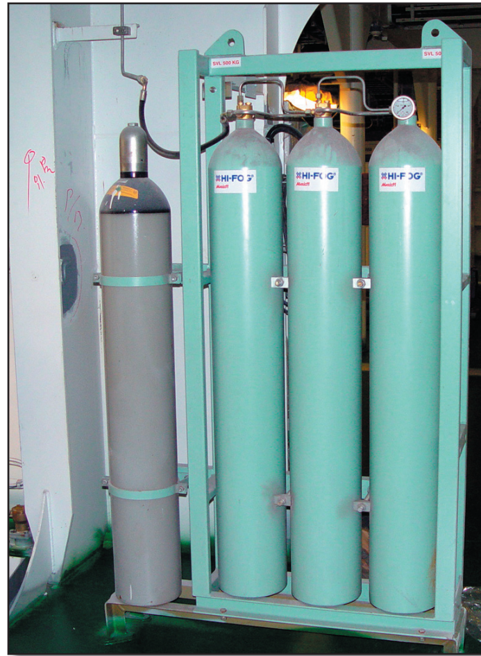
Water Mist Unit in Bosun's Store
