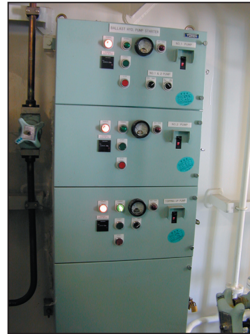
Local Starter Panel
