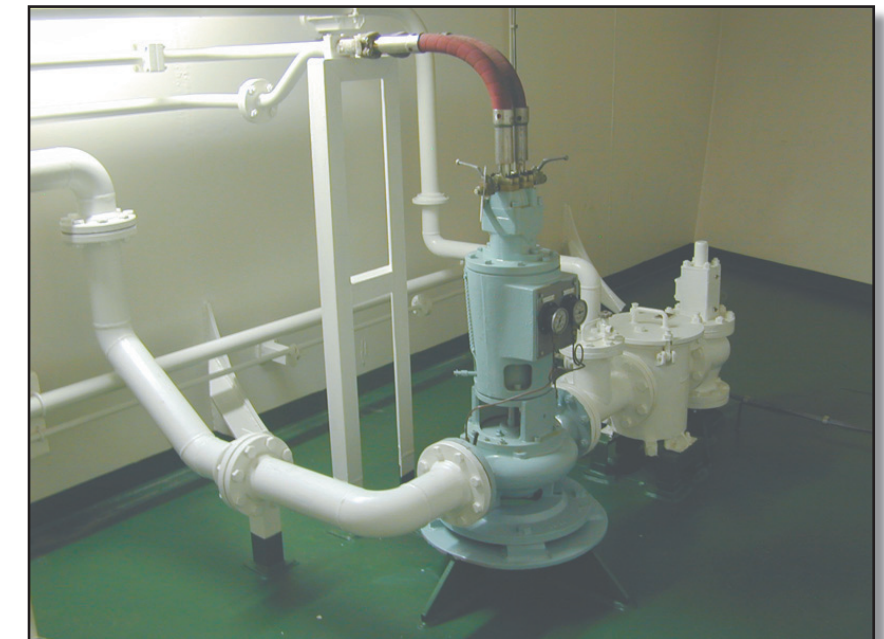
Emergency Fire Pump - Priming Pump in Forward Pump Room
