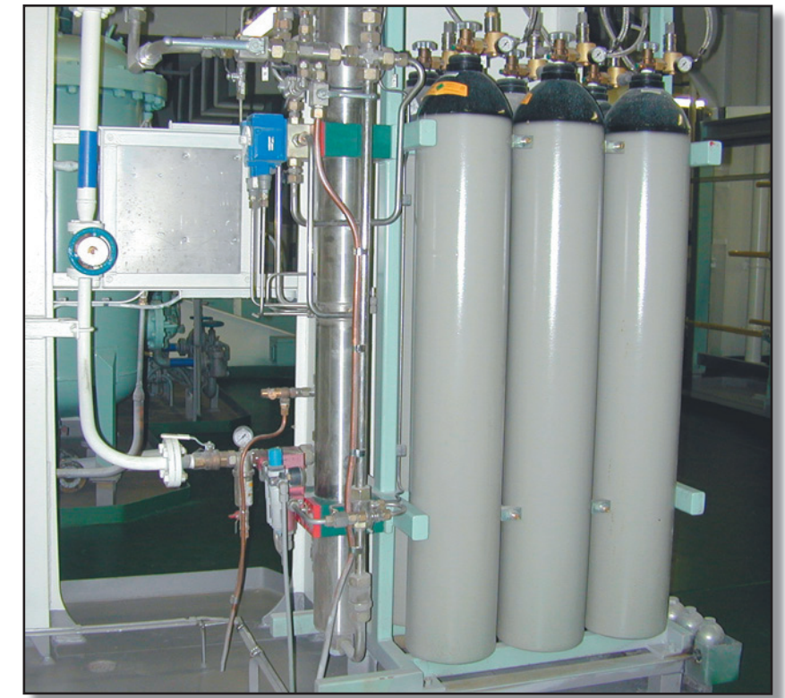
Water Mist Unit on Engine Room - Starboard Side 4th Deck
