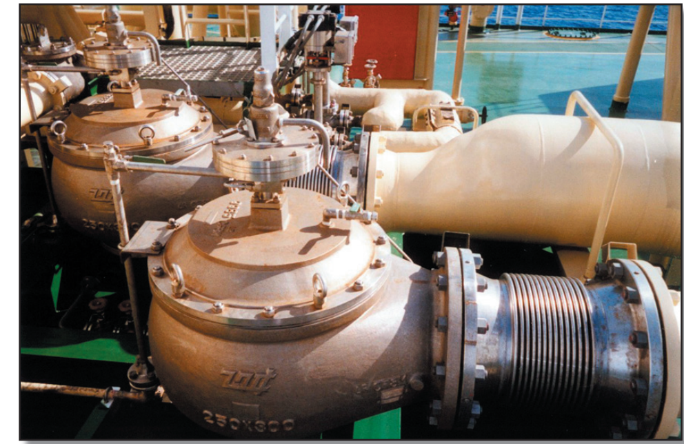
Cargo Tank Relief Valves
