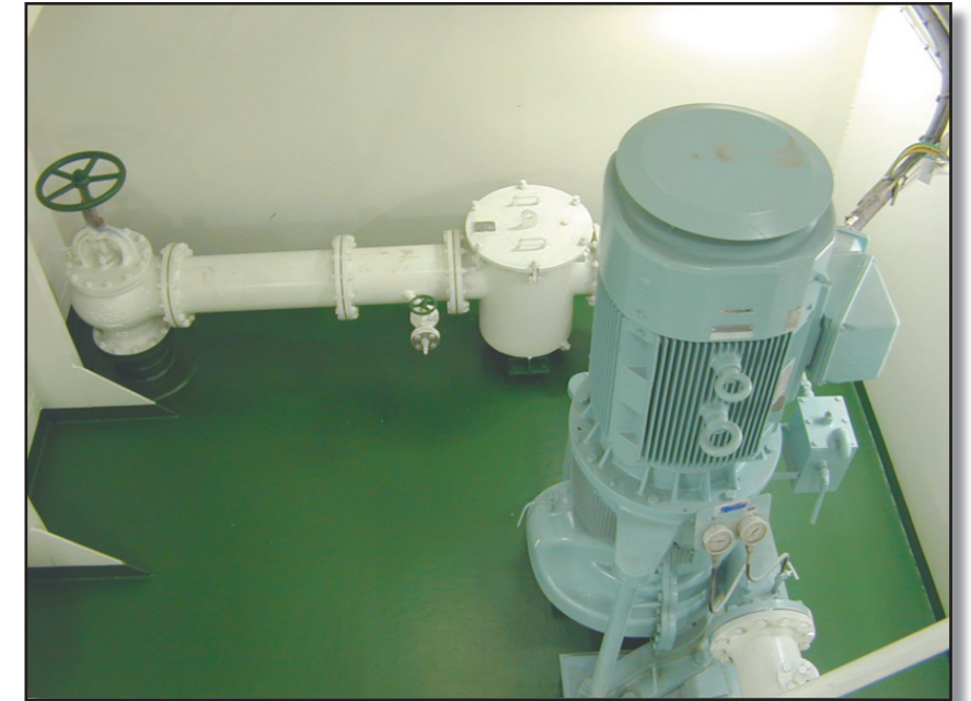
Water Spray Pump Situated in the Steering Gear Room
