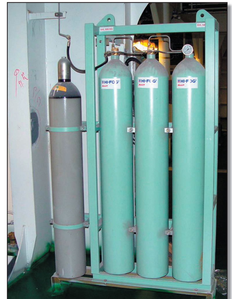
Water Mist Unit in Bosun's Store
