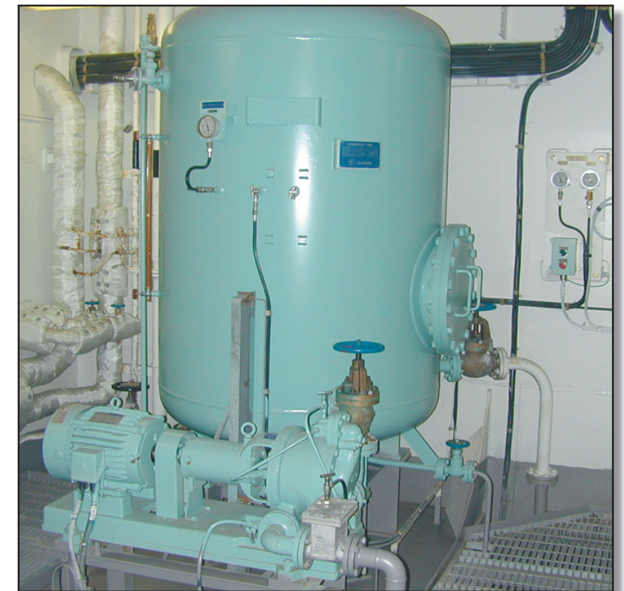
Engine Room Fire Jockey Pump and Hydrophore Tank
