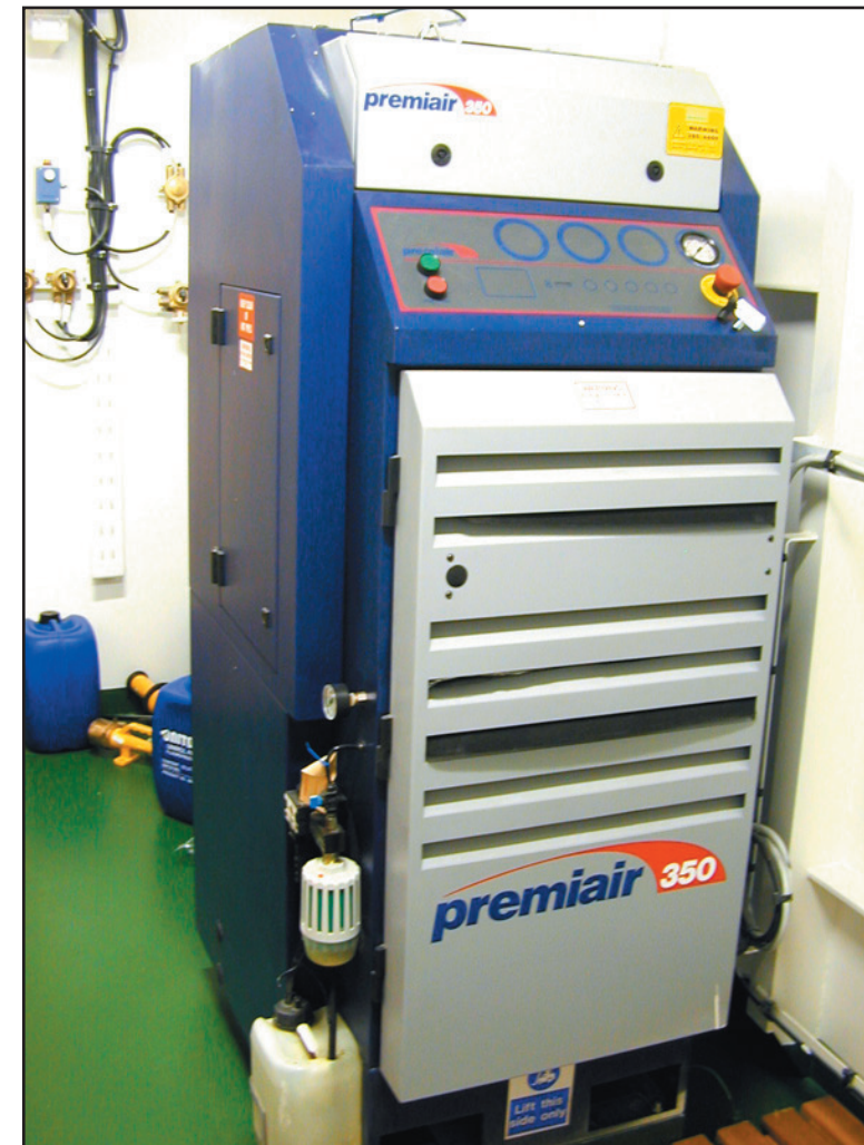
SCABA Air Compressor in Safety Equipment Locker Upper Deck Port Side
