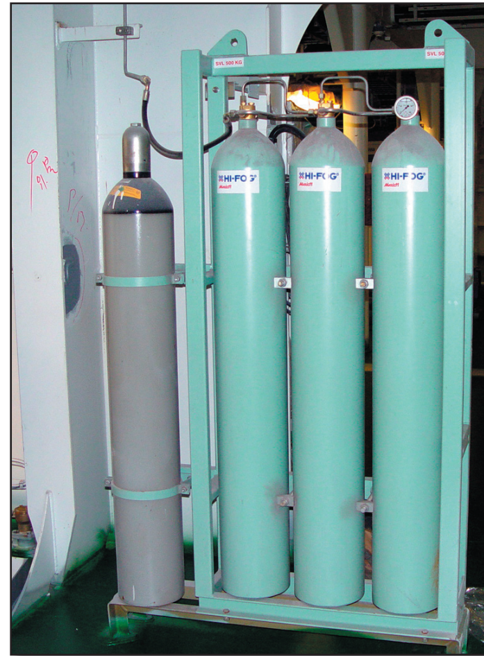
Water Mist Unit in Bosun's Store
