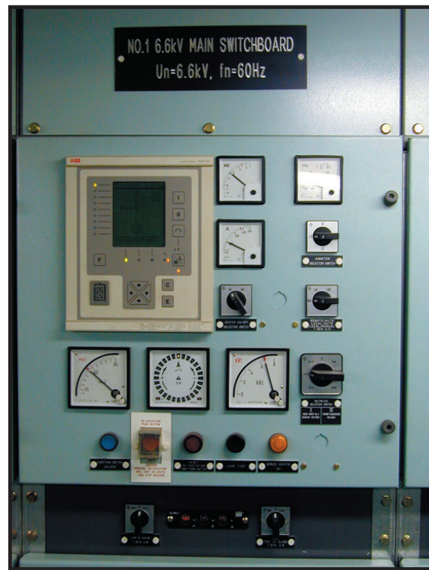
Turbine Generator PMS Panel
