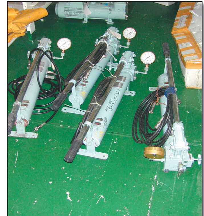
Emergency Hydraulic Pumps Situated in the Workshop
