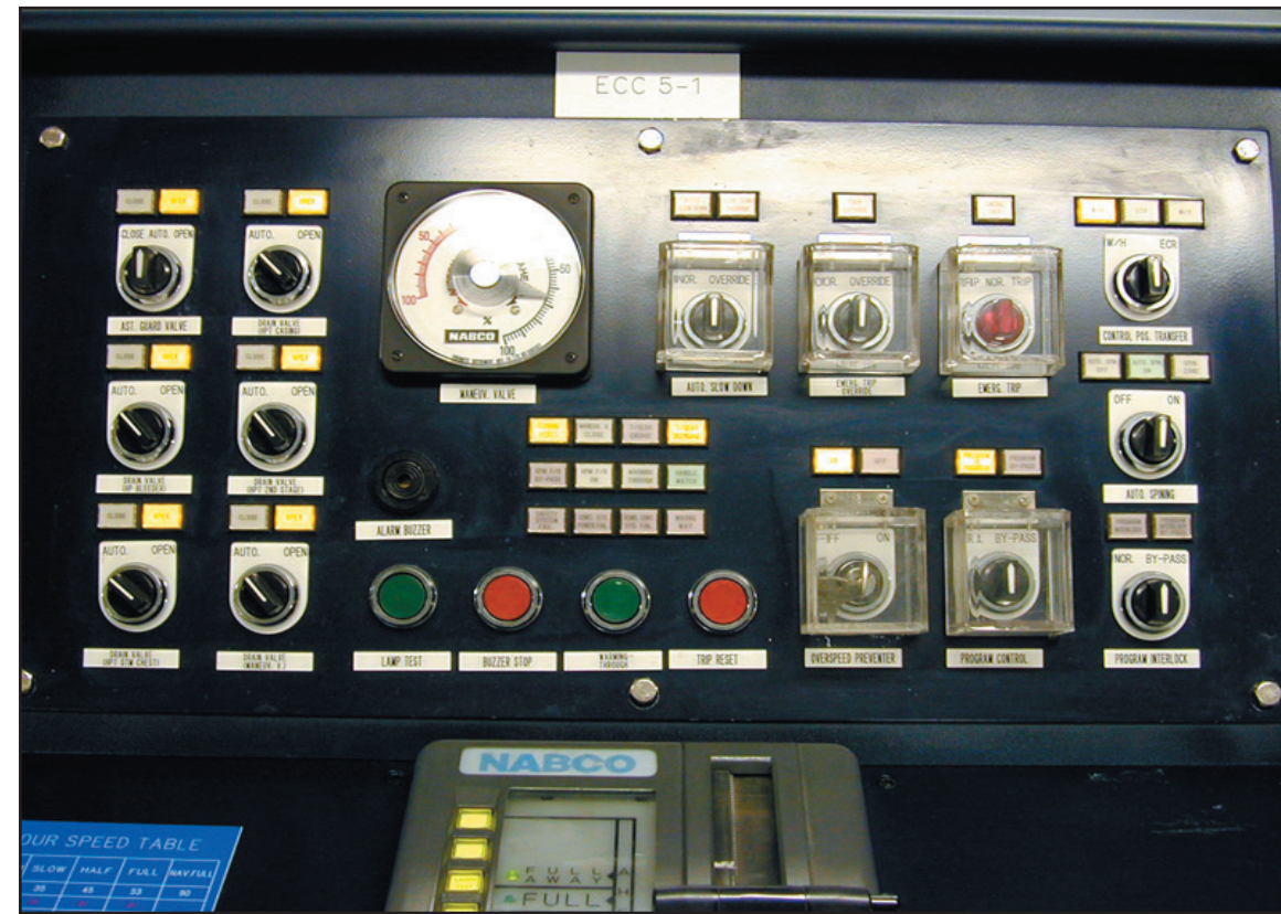
ECR Main Turbine Control Console showing Bypass Switches
