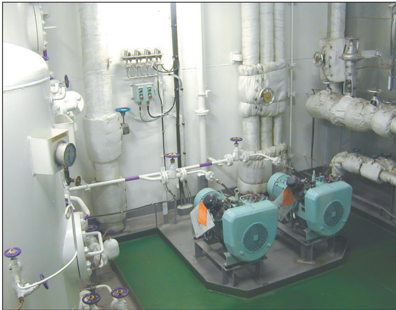
Diesel Generator Starting Air Compressors
