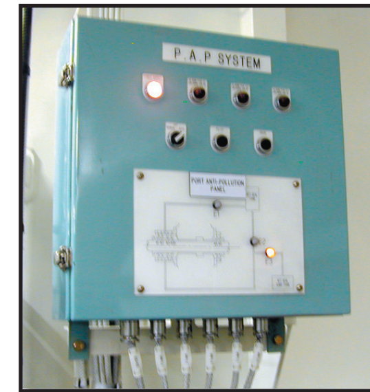
PAP Panel Situated Port Side of Shaft Tunnel
