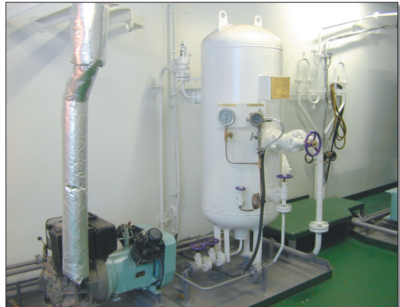
Emergency Generator Starting Air Compressors
