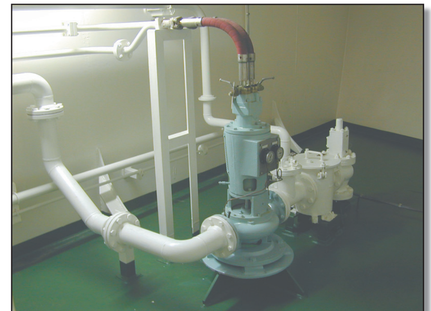
Emergency Fire Pump - Priming Pump in Forward Pump Room
