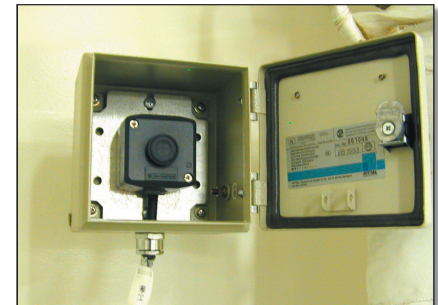
Water Mist System Local Operating Pushbutton
