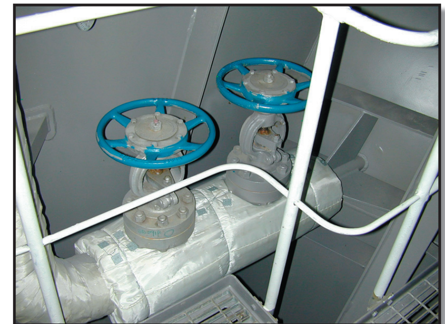
Port Boiler Blowdown Valves on Engine Room Floor Level
