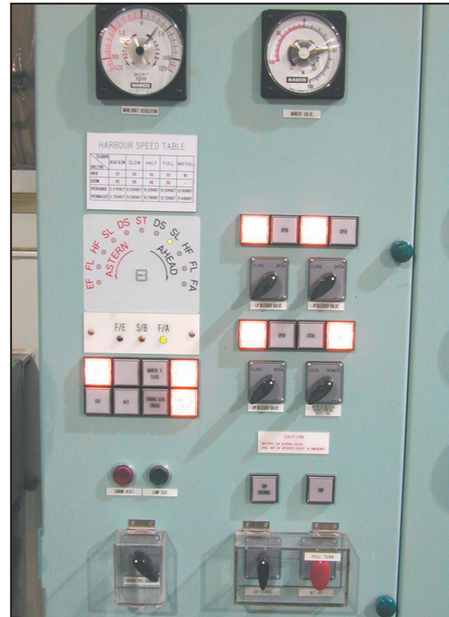
Main Turbine Emergency Control Panel
