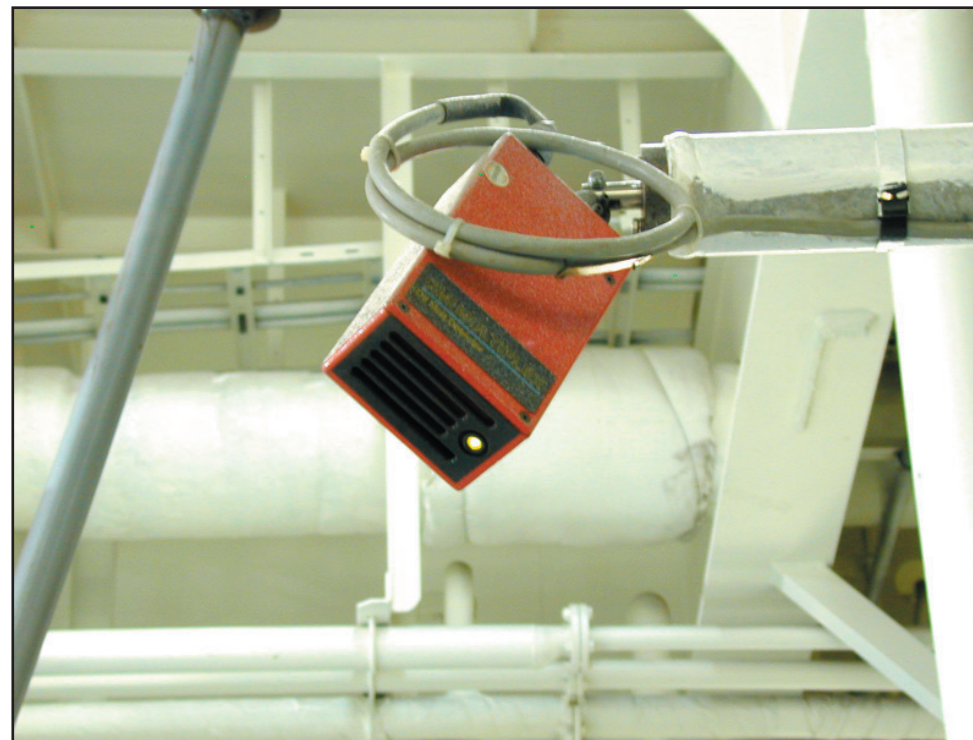
Oil Mist Detector Head above Main Turbine
