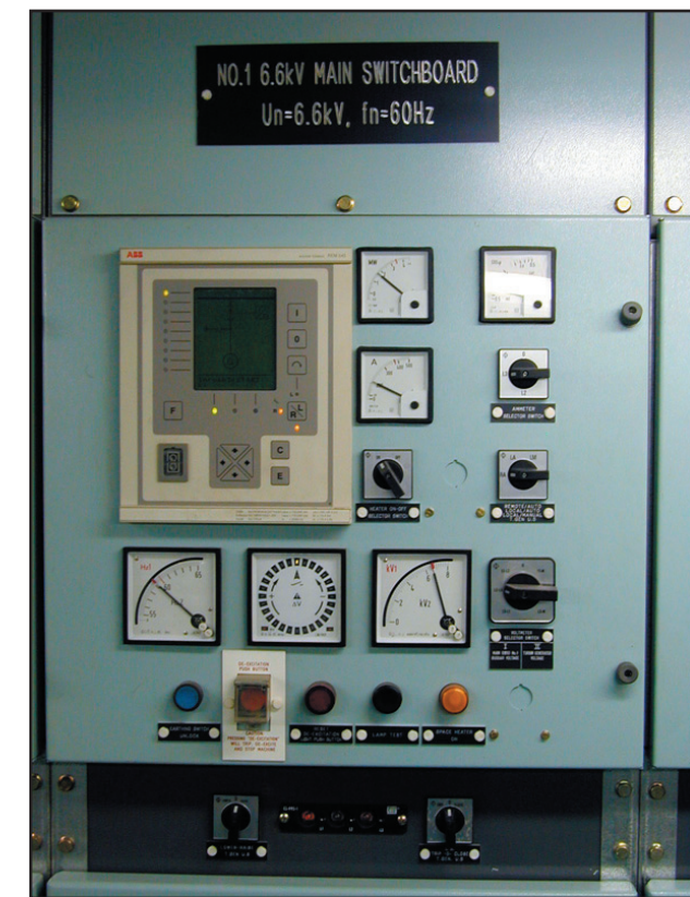
Diesel Generator PMS Panel
