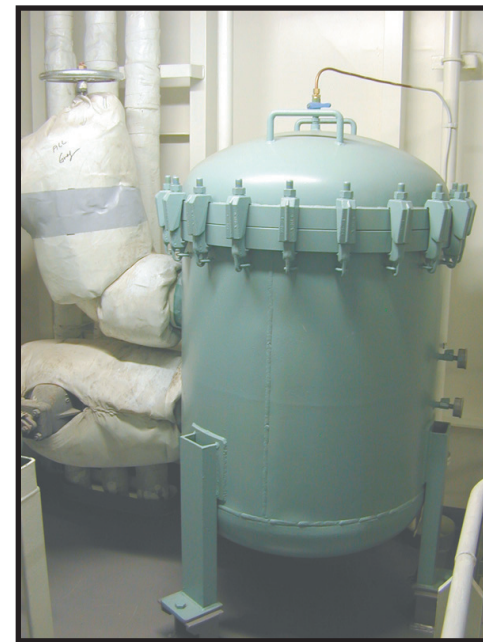
Main Feed Water Magnetic Filter
