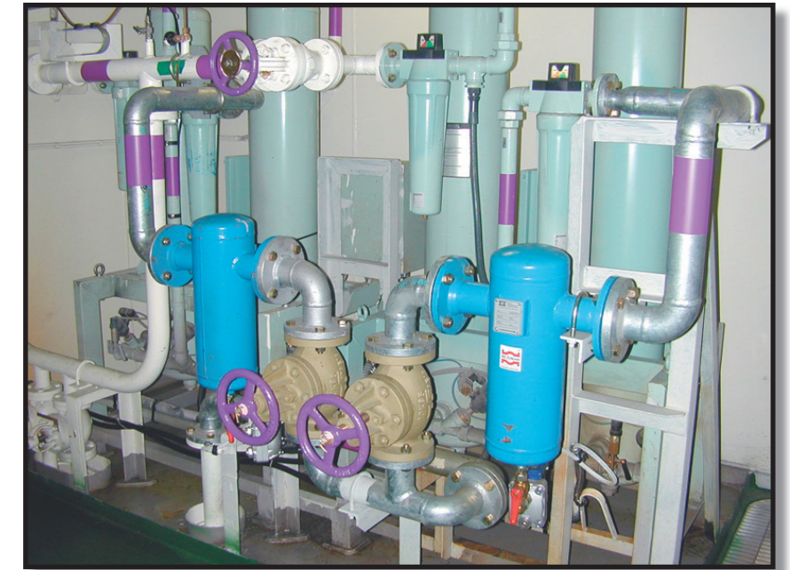
Control Air Dryers
