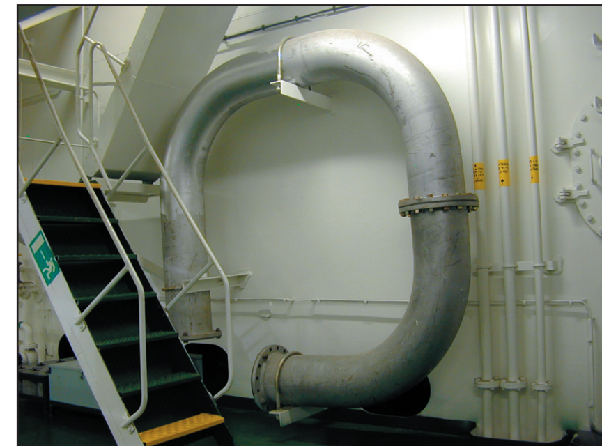
HP Turbine Emergency Piping G
