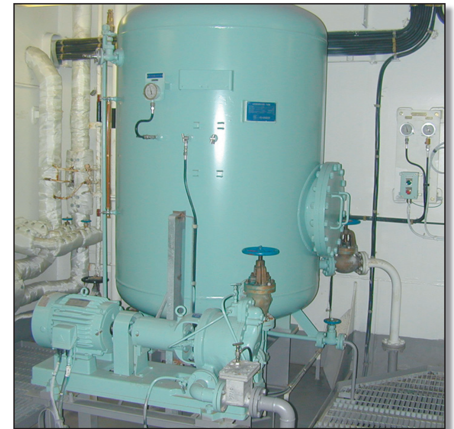
Fire Jockey Pump and Hydrophore Tank
