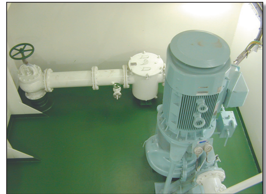
Water Spray Pump Situated in Steering Gear Room
