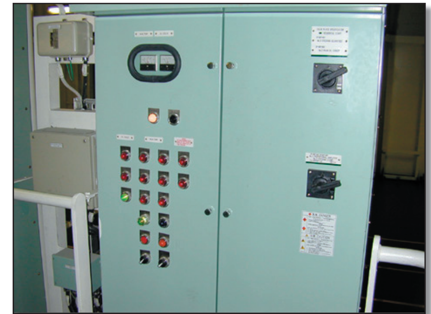
Control Panel and Proportional Amplifier Switch
