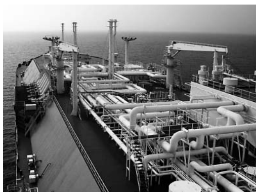
Fig. 5 Arrangement of piping on deck
