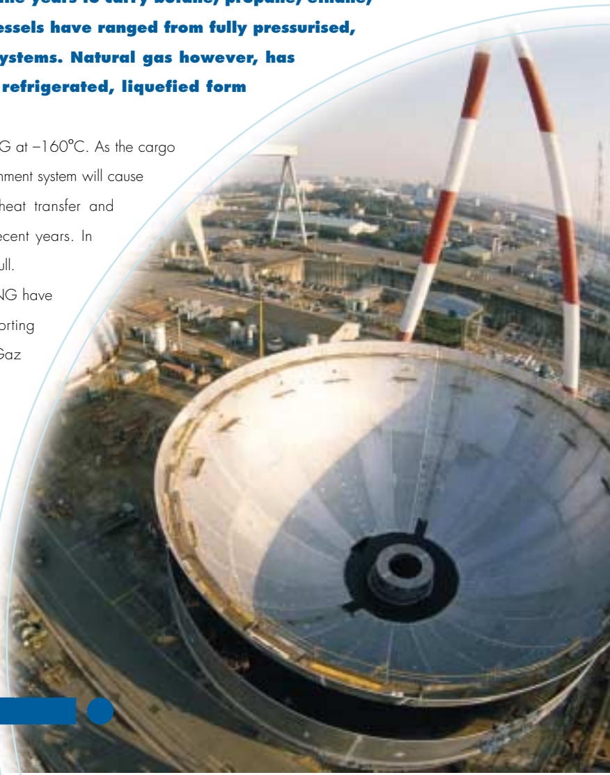
LNG tanks under construction at Mitsui Shipyard, Chiba, Japan. The tanks have been installed on LNG carriers for the North West Shelf project in Australia
